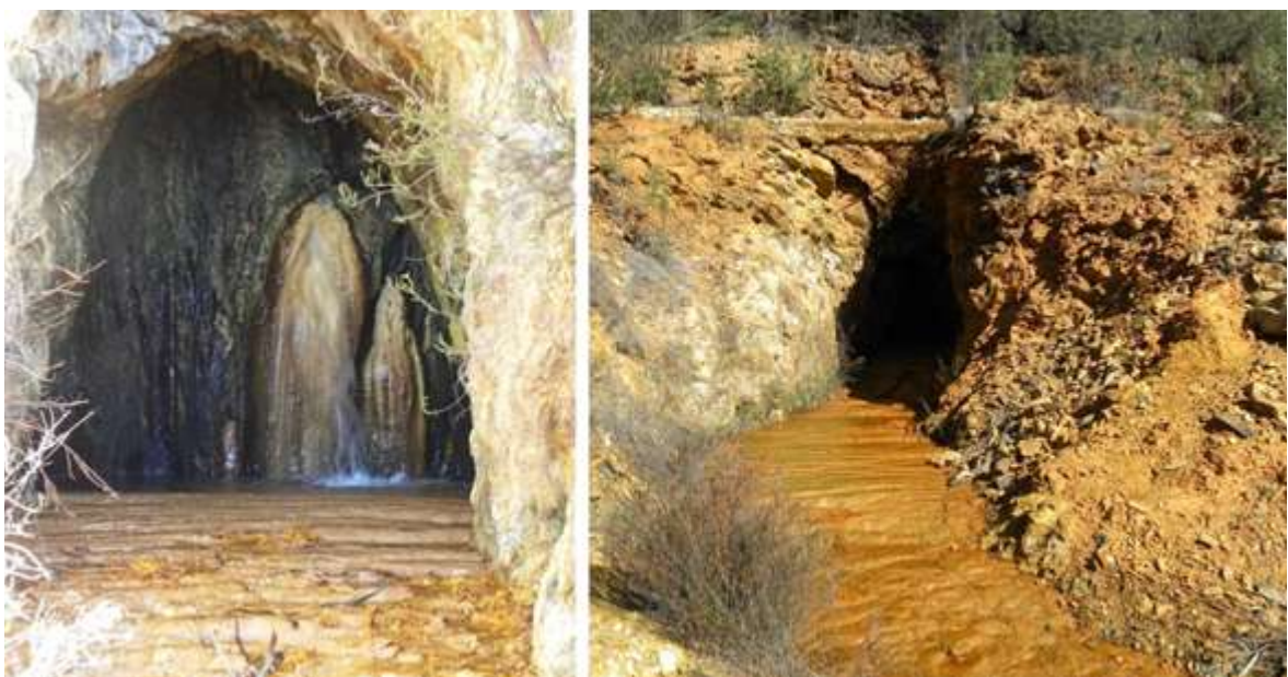
Figure 7.7: Photo of the concrete plug at the Tinto Santa Rosa mine gallery showing the leakage of highly-pressure AMD. General view (right) and detailed view (left).
