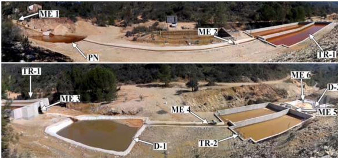
Figure 7.23: Aerial image of the passive treatment system at Esperanza Mine; water flows from upper left side of the figure and outflows from the lower left side.
