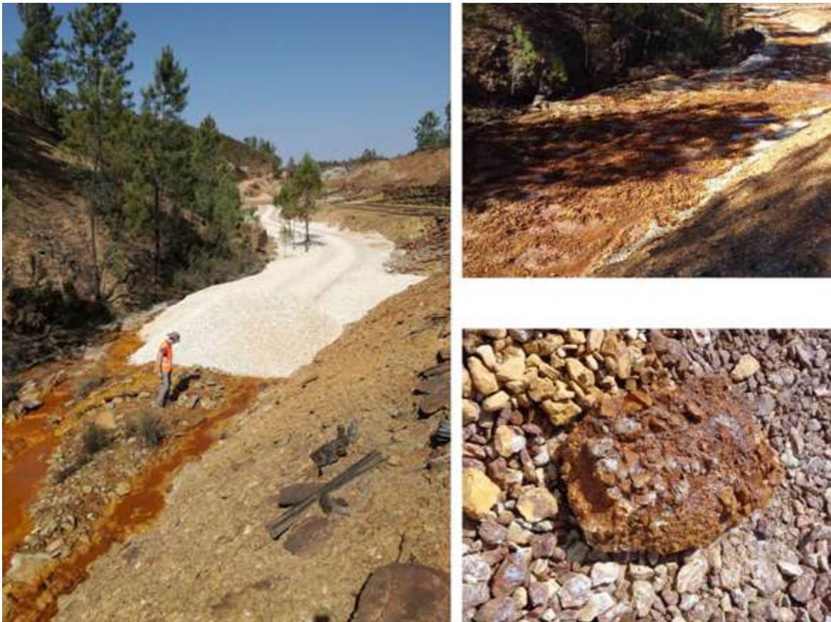
Figure 7.18: Construction of an Open Limestone Channel (OLC) after the accidental mining spill of La Zarza (June 2017) due to the break of a concrete plug (left). This system failed to treat the spilled AMD due to limestone grains coating due to intense Fe precipitation. It can be seen the coating of the channel and a limestone block totally coated by Fe precipitates (right).
