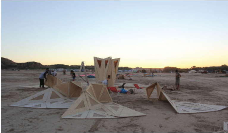
Fig. 2 Construction on site of the Nomad Folding Flax Pavilion erected in the desert of Monegros, Zaragoza. Photo by Ji Won Jun (2017)
